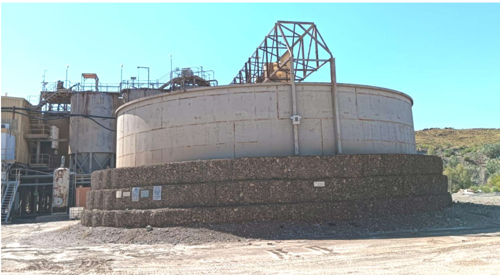
Bamboo Creek Processing Plant Thickener.
